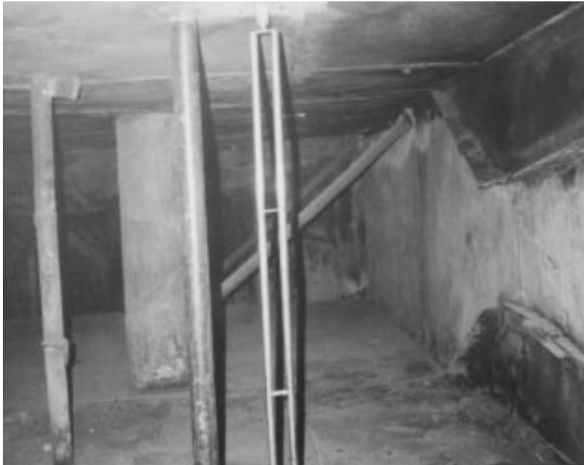
Figure 11 Secondary Air Flow Measurement
