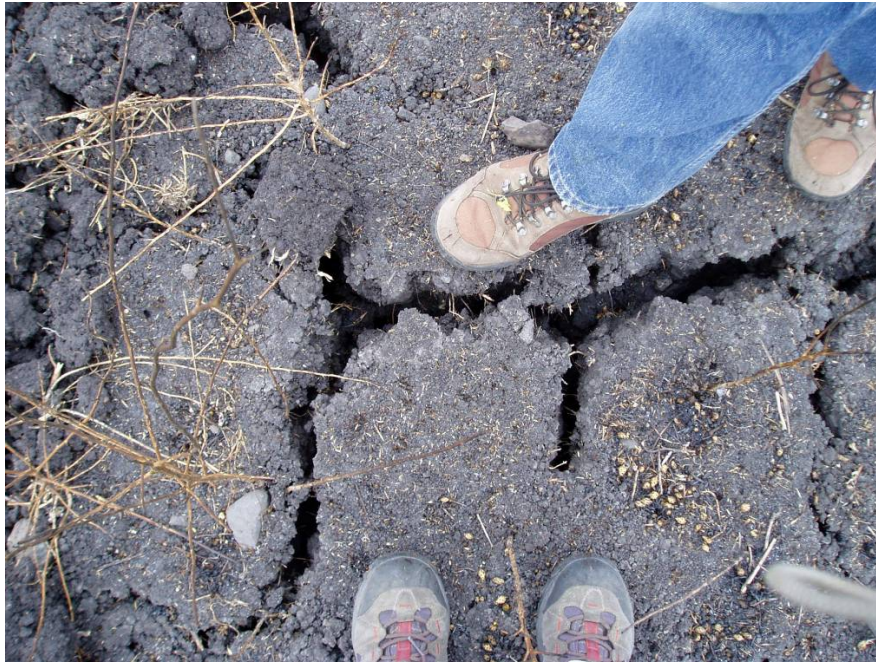
Figure 4. Large cracks developed in Clear Lake clay on the southern half of the site.
